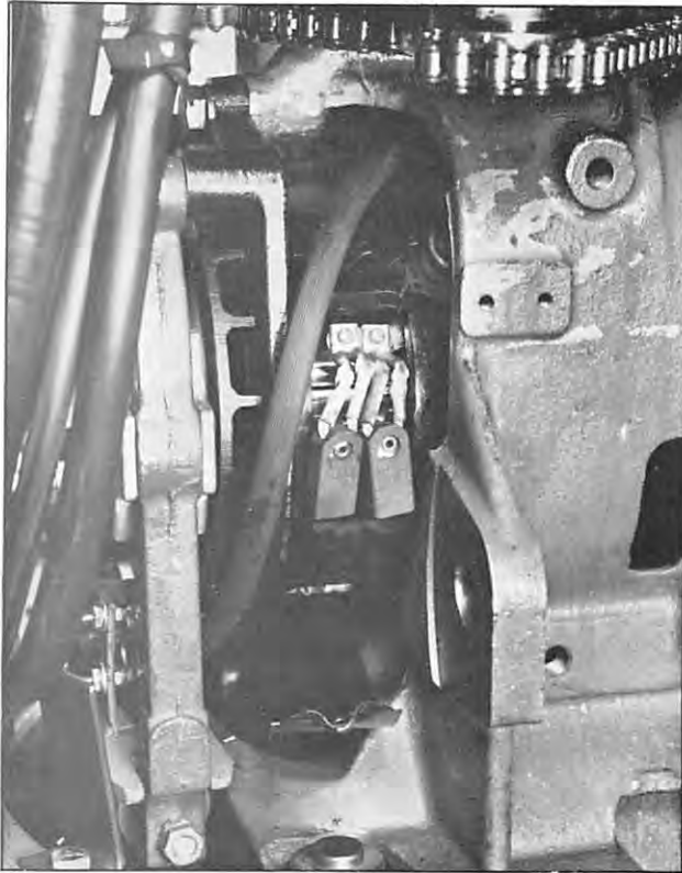
Plate 7518. Typical Drive Motor
